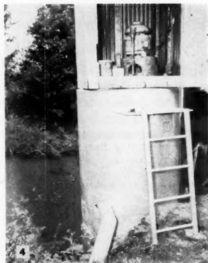
Fig. 4. River pump, a half mile from the gas station is installed in a concrete pit and protected from the weather by a steel shed.
